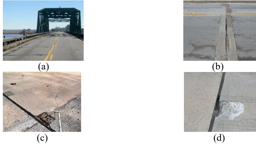
Fig. 1. Deck elements of Bridges #1-4: (a) approach (b) pourable joints (c) and (d) deck joints (GDOT, 2022).
