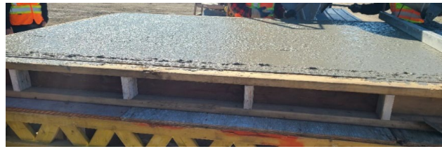
Fig. 3. Levelling of the Dura ® ECC mix on 2% slope (Left Side is low end)
