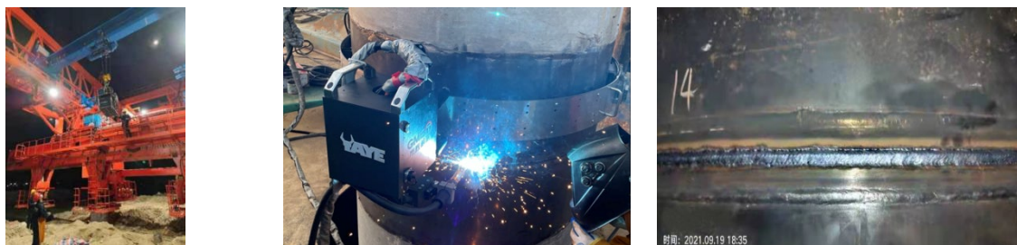
(a) a pile-beam integrated (PBI) machine with a welding robot (b) welding process of bridge pipe pile (c) the appearance of the weld
