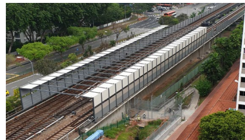
Fig. 3(b). Typical 5m Height Portal Type Noise Barriers at Track Turnout
