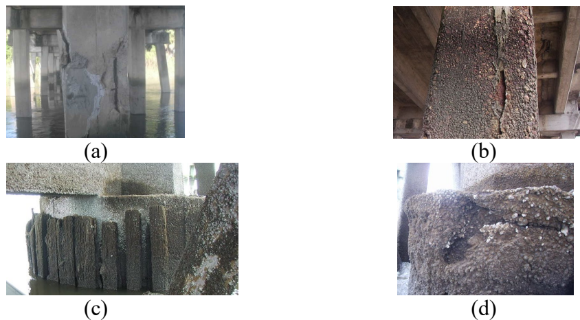
Fig. 3. Substructure elements of Bridges #1-4: (a) RC pile; (b) RC pile; (c) column; (d) pile cap deteriorated (GDOT, 2022).
