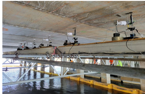
Fig. 2. Overall view of instruments on the scaffolding
