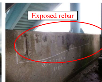
Fig. 7. Deterioration of T-bridge
